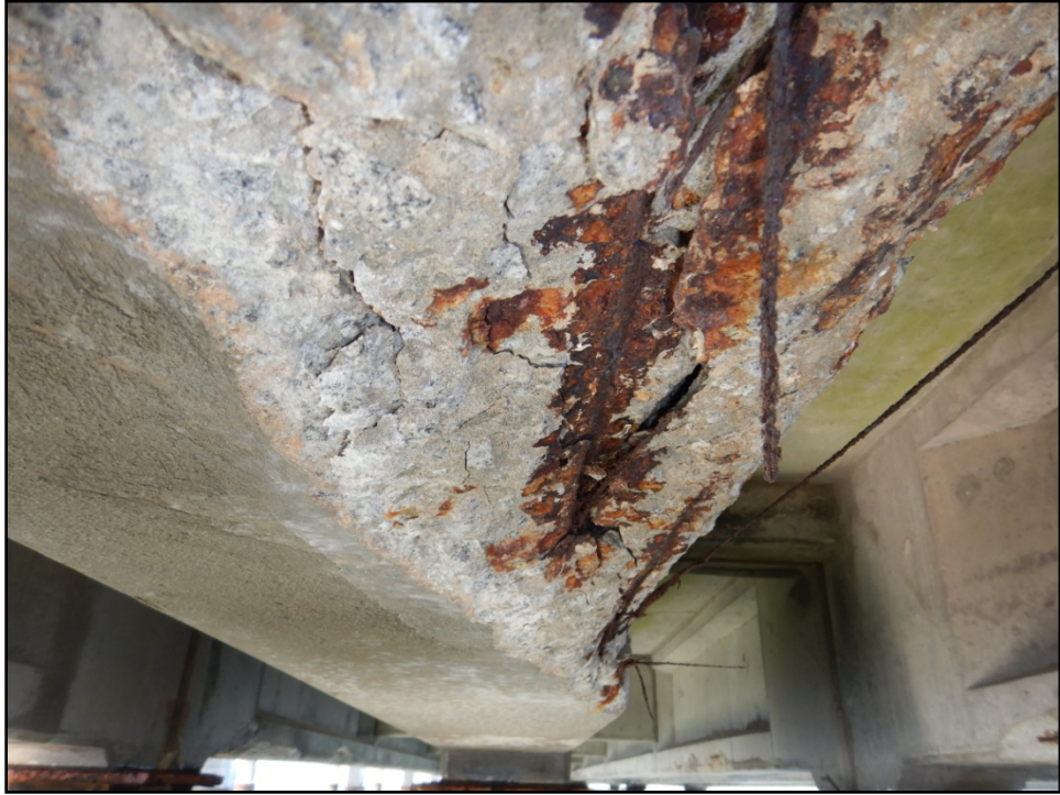
Photograph 10: Typical Increased Deterioration on Prestressed Concrete Beam
