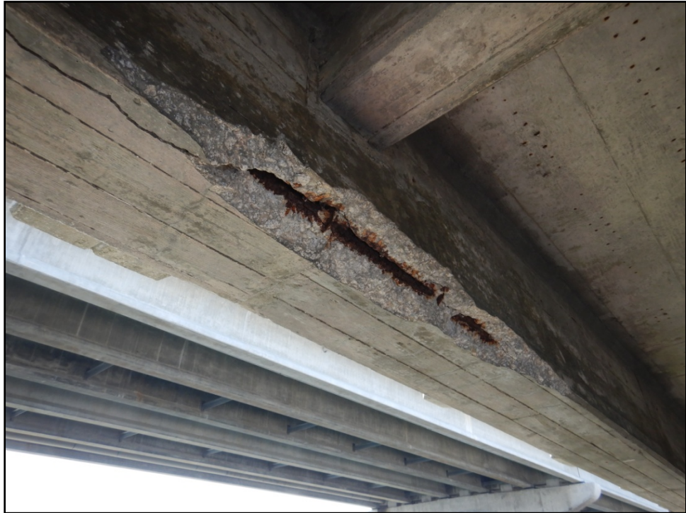
Photograph 11: Typical Increased Spalling on Reinforced Concrete Beam
