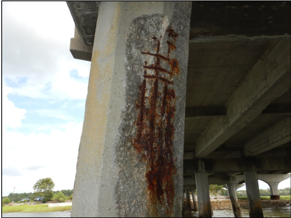
Photograph 16: Spall Not Previously Noted at Pile 27A
