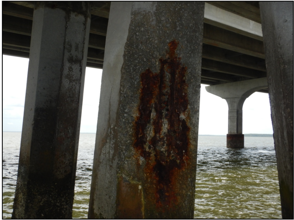
Photograph 15: Spall at Pile 23E
