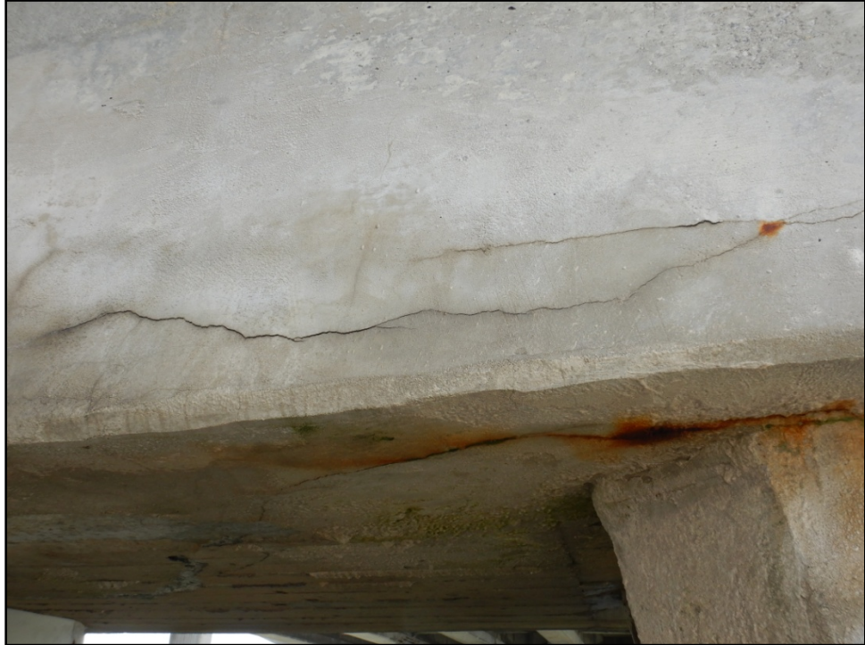
Photograph 13: Typical Crack with Rust Staining in Pile Cap
