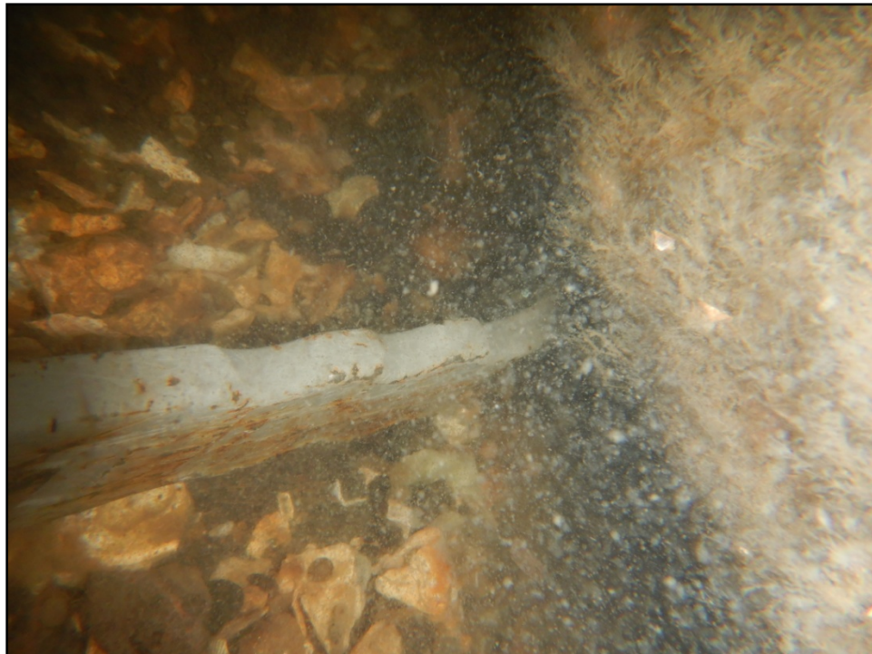
Photograph 20: Typical Pile Undermining, Bent 7
